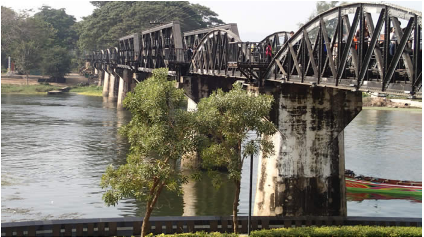
Same view today with the missing two curved spans replaced by rectangular ones - and the shrapnel gouges patched.
